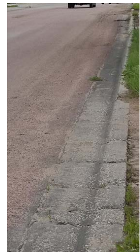
Curb with the rating of fair.
