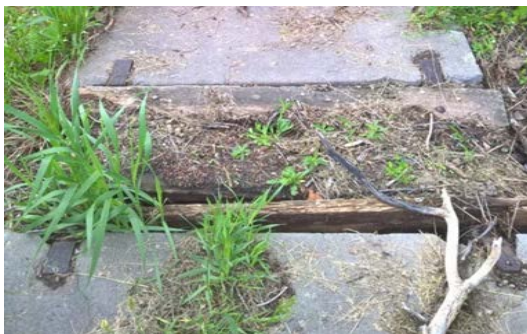
Dangerous – Church Avenue & 10 th Street
