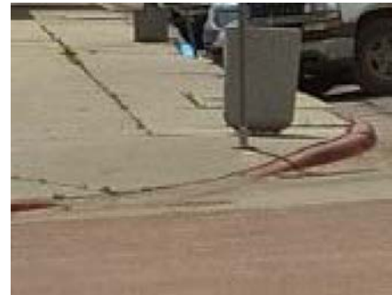
No ADA Warning Panel – Main Street & 6 th Street
