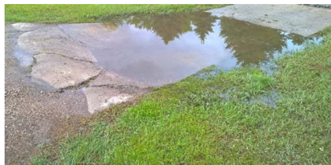
Drainage issue across driveway.
