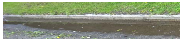
Curb with the rating of poor.
