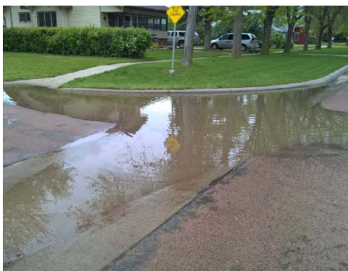
Drainage issue on 10 th Street and Felton Avenue
