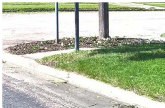
No Ramp – Church Avenue & 6 th Street
