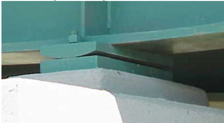
Figure 13.8 Rocker Bearing with nut over tightened
