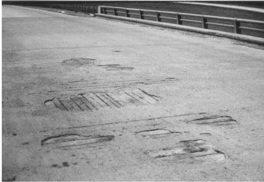
Figure 7.19 Scaling of Concrete due to Improper Clear Cover of Reinforcement
