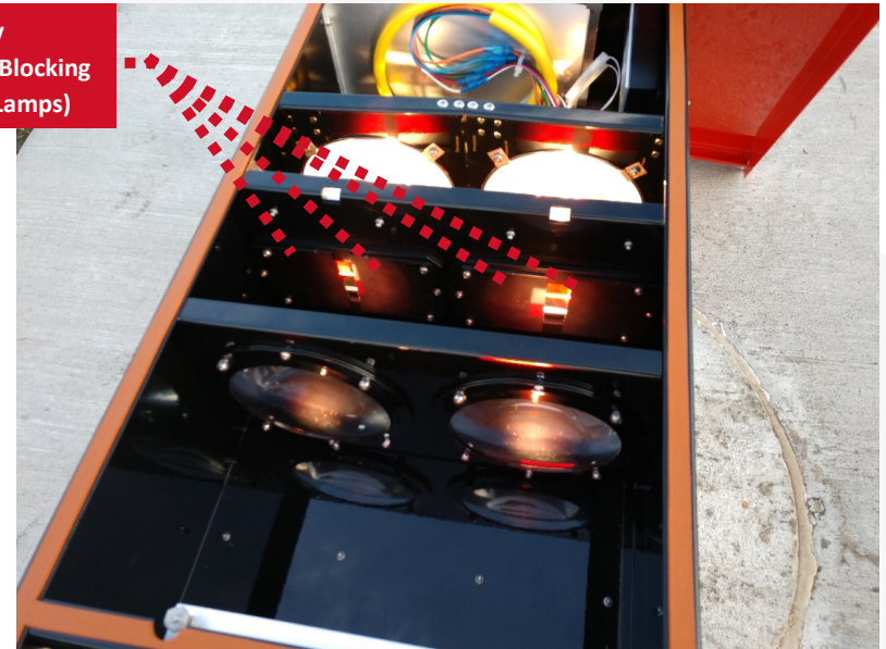
Baffles Incorrectly Installed In PAPI
