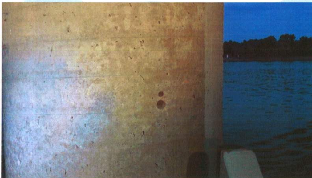
Photo 6 - Bent 5, Unpatched Chloride Test Hole
