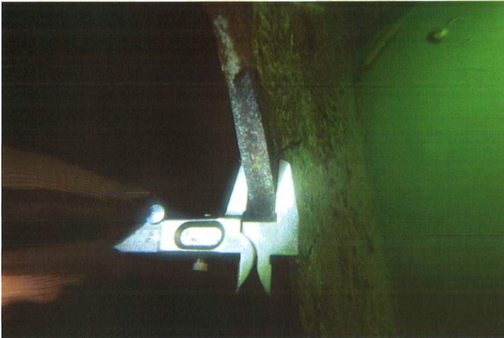
Photo 12 - Pier 7, Steel H-Pile Condition Close Up
