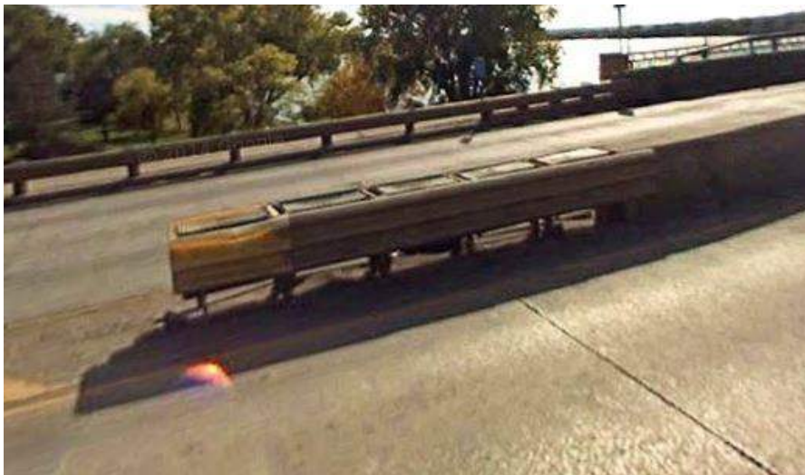
Figure 6: Crash Cushion at Eastern End of US 14 Missouri River Bridge
