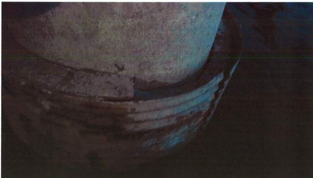
Photo 5 - Bent 4, Pile 4, Perforations and Voids in Encasement
