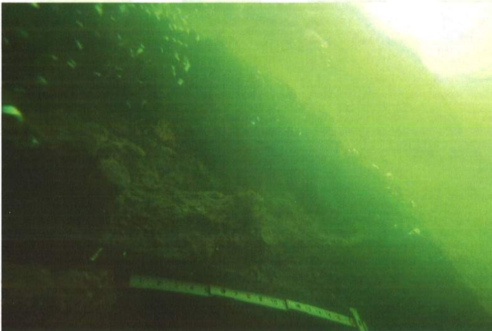
Photo 14 - Pier 8, North Face of Footing, Eposed Reinforcing Steel
