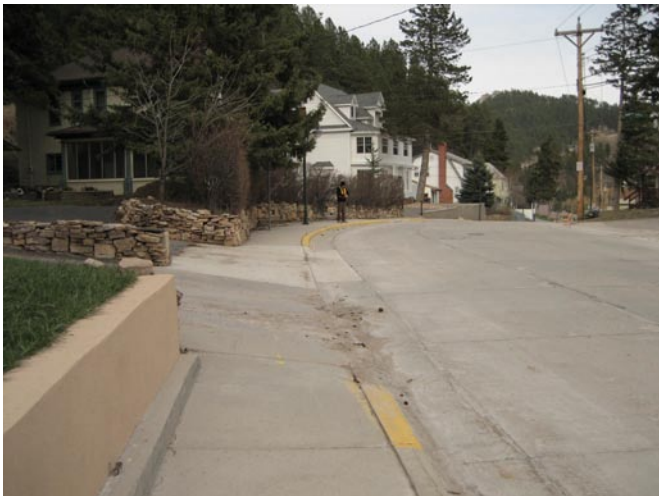
Cross-slope across driveways is a common deficiency for Deadwood sidewalks. A 36 inch wide sidewalk travel way in combination with a compound apron slope can often mitigate this type of cross slope deficiency (see sketches).
