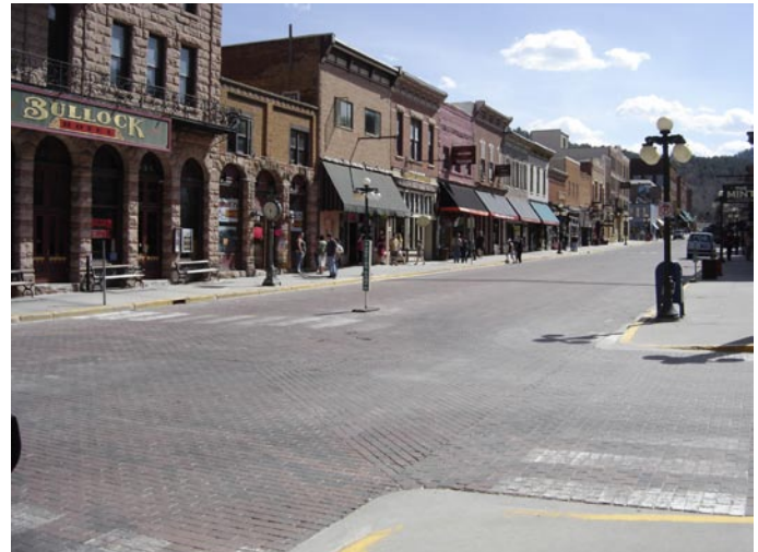
Sandy soils and the underlying brick pavers give pavement markings a short life. Markings were reapplied during the Summer of 2008.
