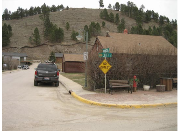
The lack of curb ramps makes an otherwise adequate sidewalk inaccessible for some users. The plan calls for the construction of 46 new curb ramps including here at the intersection of Cliff Street and Burlington Street.
