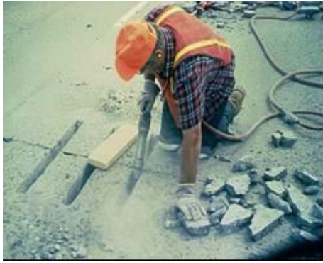
Step 1 & 2. Slot creation and material removal. Slots are cut and concrete material is removed.
