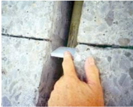
Step 5. Caulking the joint/crack. The joint/crack edges are caulked to stop the flow of material from the slot.
