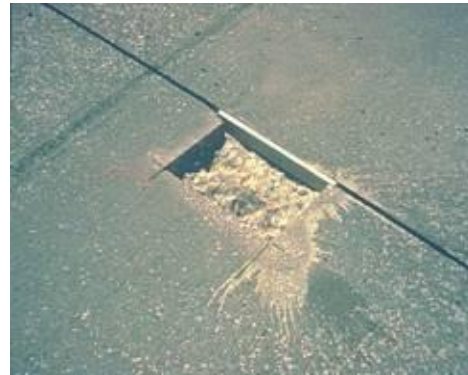
Step 4. Joint preparation. It is important to maintain the existing joint reservoir during construction.
