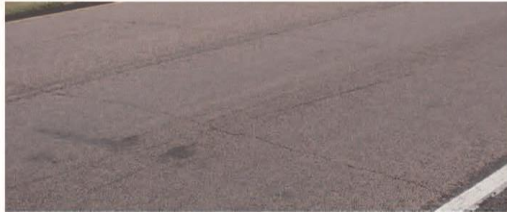
LOW SEVERITY - Crack width is less than 1/4 inch or Routed & sealed crack width less than 1/2 inch (Crack spacing is greater than 50 feet average spacing)
