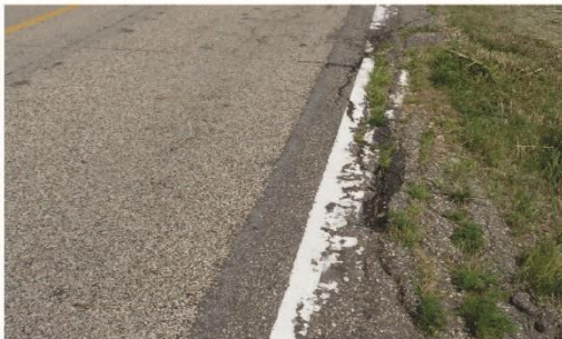
High - Cracks greater than 1/4-inch; may have loose or missing pieces or potholes or alligator cracking.
