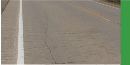
Low - Longitudinal cracking in and between wheel paths (1% to 9% of the slabs)
