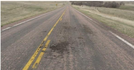
HIGH SEVERITY - Alligator pattern clearly developed with spalling and distortion (greater than 25% of the wheel path is affected.)
