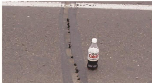
HIGH SEVERITY - Crack width greater than 1 inch or crack width is greater than 1/4 inch and Depression caused by crack is greater than 1/4 inch (Crack spacing is less than 25 feet and greater than 12 feet average spacing)
