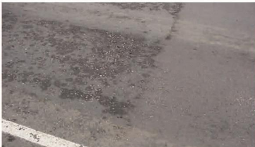
High - Sections greater than one square foot may be pitted, stripped or eroded away.
