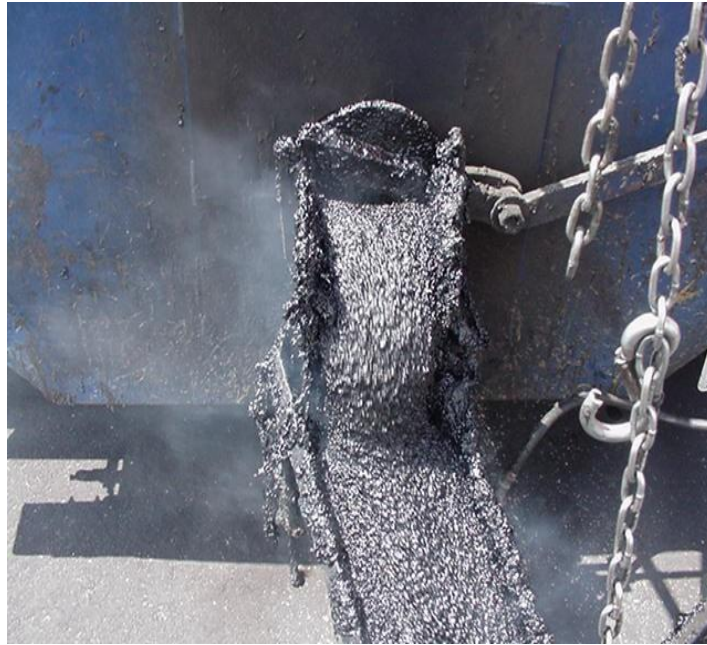
Step 1. Hot kettle equipped with chute facilitates placement across the joint prior to striking the material level with a squeegee.
