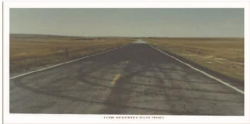
LOW SEVERITY - Patch shows no visual distress with a smooth ride (1% to 9% of the section is affected)
