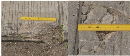
HIGH SEVERITY JOINT SPALLING - Spalls greater than 6 inches wide and may have significant loss of material (25% to 49% of the joints are affected)
