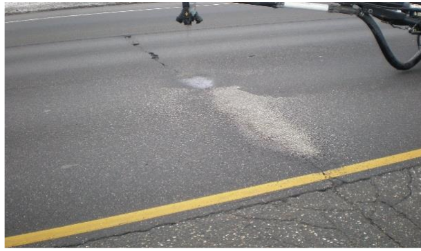
Step 4. Cover aggregate is used to protect the patch as the emulsion cures.
