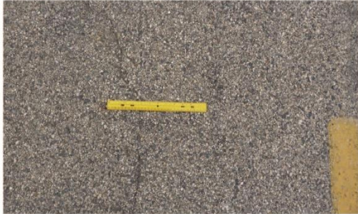
Low - Hairline crack(s) running parallel to centerline.
