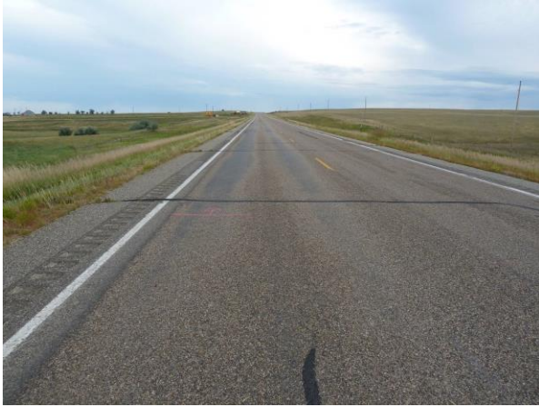
Step 1. Rutted pavement.
