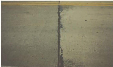
Medium - Seal damage to 10% to 50% of the joint (10% to 24% of the joints are affected)
