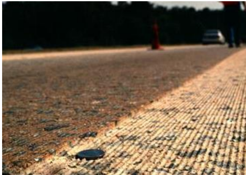
Step 2. Diamond grinding depth. Generally, roughly \frac{1}{4} inch of the surface is removed in a single pass.
