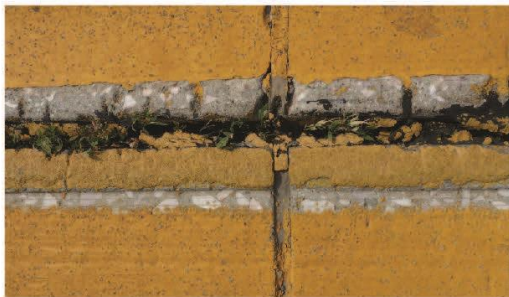
High - Seal damage to greater than 50% of the joint (25% to 49% of the joints are affected)
