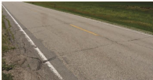
MEDIUM SEVERITY - Crack width is greater than 1/4 inch and less than 1 inch and/or Depression caused by crack is less than 1/4 inch (Crack spacing is less than 50 feet and greater than 25 feet average spacing)
