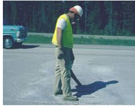
Step 3 & 4. Sandblasting and cleaning. Slots are sandblasted and cleaned in preparation for dowel bars.
