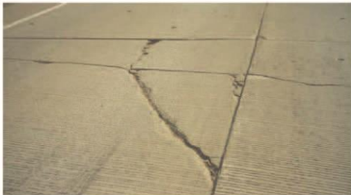
HIGH SEVERITY - Crack is spalled, and/or faulted greater than 1/2" and/or piece is broken (25% to 49% of the slabs)
