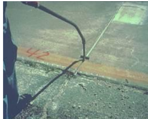
Steps 7 & 8. Curing & joint sealing. The final steps include texturing and providing adequate curing.
