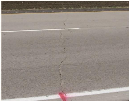
High - Transverse cracks greater than 1/4-inch wide extending the full width of panel.
