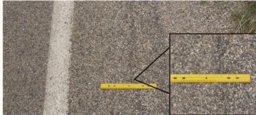
Low - Hairline cracks just beginning to show; random with no pattern; may be up to 1/8-inch wide.
