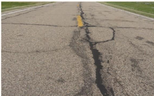
High - Single cracks are wider than 1/8-inch.
