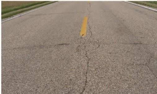
Moderate - Cracks parallel to centerline are about 1/8-inch wide.
