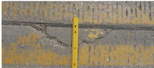
MEDIUM SEVERITY - Spalls 3 to 6 inches wide and may have loss of material (10% to 24% of the joints are affected)
