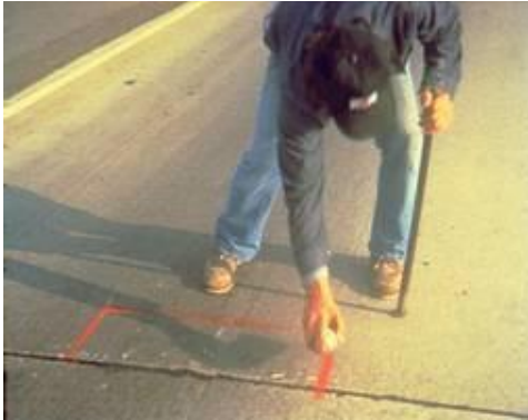
Step 1. Repair boundary marking. Determine extent of unsound material, and mark repair boundaries.
