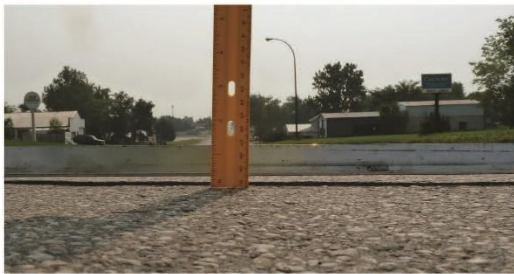
Moderate - Wheel path depressions of 1/4-inch to 1/2-inch
