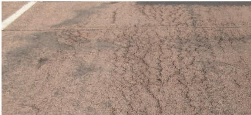
MEDIUM SEVERITY - Alligator pattern clearly developed (10% to 24% of the wheel path is affected)
