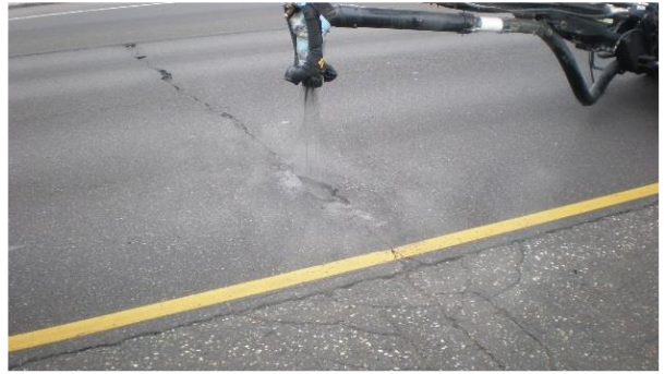
Step 2. The blow patch truck begins spraying a slurry of aggregates and emulsion into the pothole.
