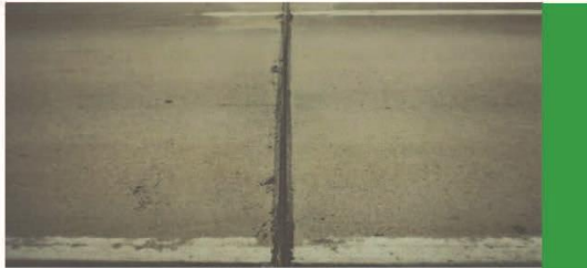
Low - Seal damage to less than 10% of the joint (1% to 9% of the joints are affected)
