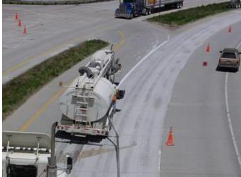
Step 1. Multiple passes of the grinding equipment are used to remove material from the pavement surface.
