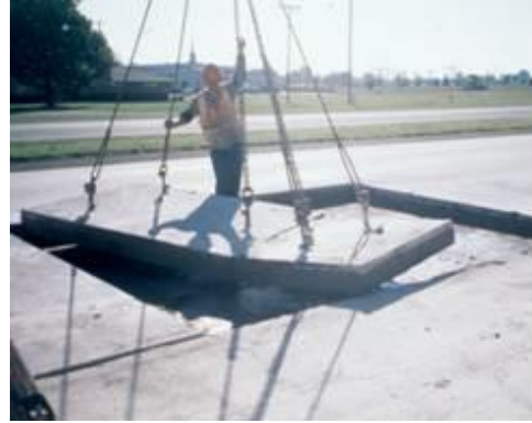
Step 2. Concrete removal. Removal of slab material is best accomplished using the lift-out method or by breakout.
