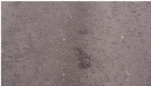
Moderate - Some aggregate loss; small areas may be stripped away.
