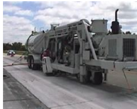
Steps 8 & 9. Diamond grinding & joint sealing. Final steps often consist of diamond grinding and joint sealing.
