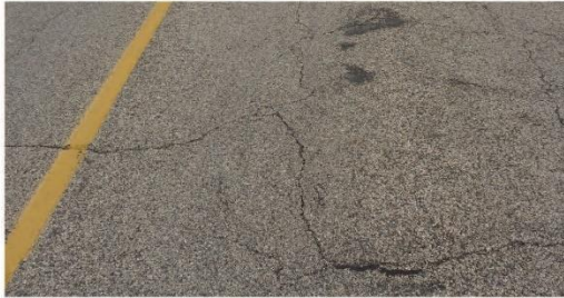
LOW SEVERITY - Fine parallel cracks in the wheel path (1% to 9% of the wheel path is affected)
