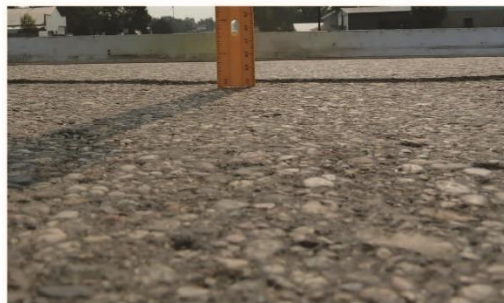
High - Wheel path depressions greater than 1/2-inch.
