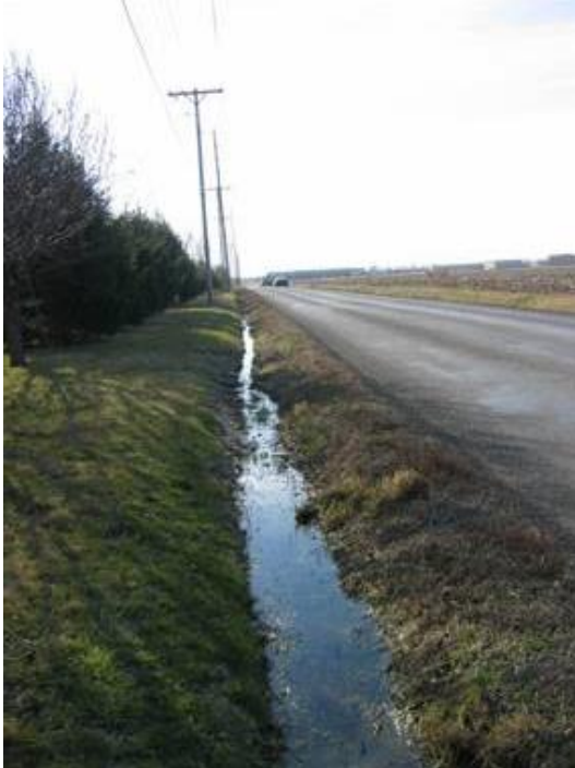
(a) Ditch with obstructed flow.
