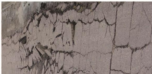
High - Shoving and major changes in pavement profile that require vehicles to slow from normal speeds.
