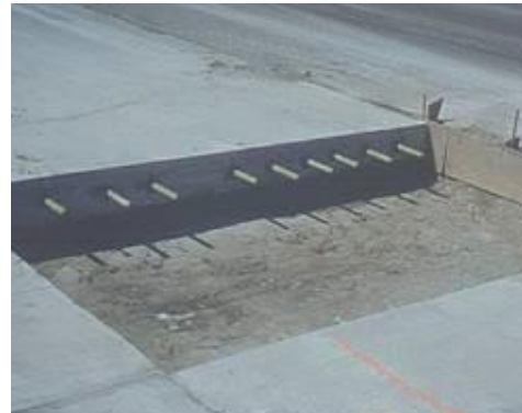
Step 4. Load transfer provision. Proper restoration of load transfer should be considered.
