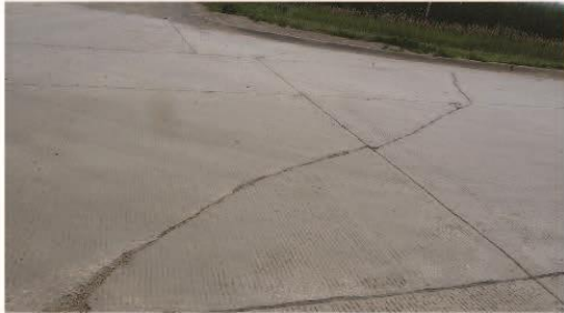
MEDIUM SEVERITY - Crack is spalled slightly, and/or faulted less than 1/2", or piece broken with tight crack
