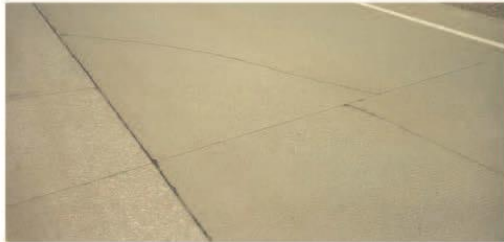
LOW SEVERITY - Crack is not spalled with no faulting & piece is not broken (1% to 9% of the slabs)
