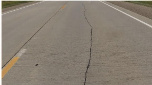
Medium - Longitudinal cracking between wheel paths (10% to 24% of the slabs)
