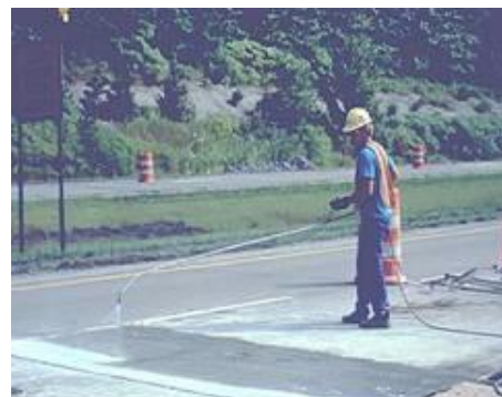
Steps 6 & 7. Texturing & Curing. The final steps include texturing and provide adequate curing.
