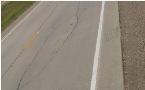
High - Longitudinal cracking in wheel paths (greater than 49% of the slabs)
