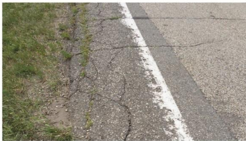
Moderate - Cracks 1/8 to 1/4-inch located 1-2 feet from the edge of the road; may have an alligator pattern.
