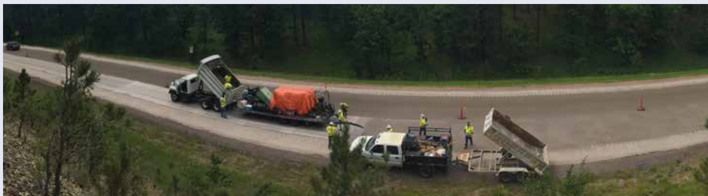
A high-friction surface treatment being added to a Black Hills highway curve in 2017
