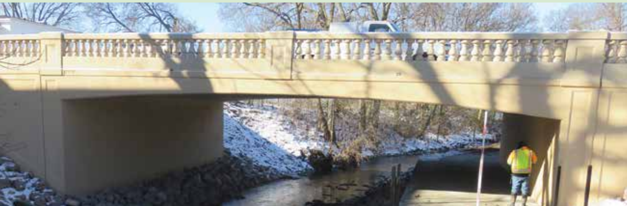
The spindle railings on the new Pine Street bridge over Marne Creek in Yankton echo the design of the century-old structure it replaced. The city of Yankton paid more than the required 20% in matching funds for the enhanced aesthetics of the new structure.
