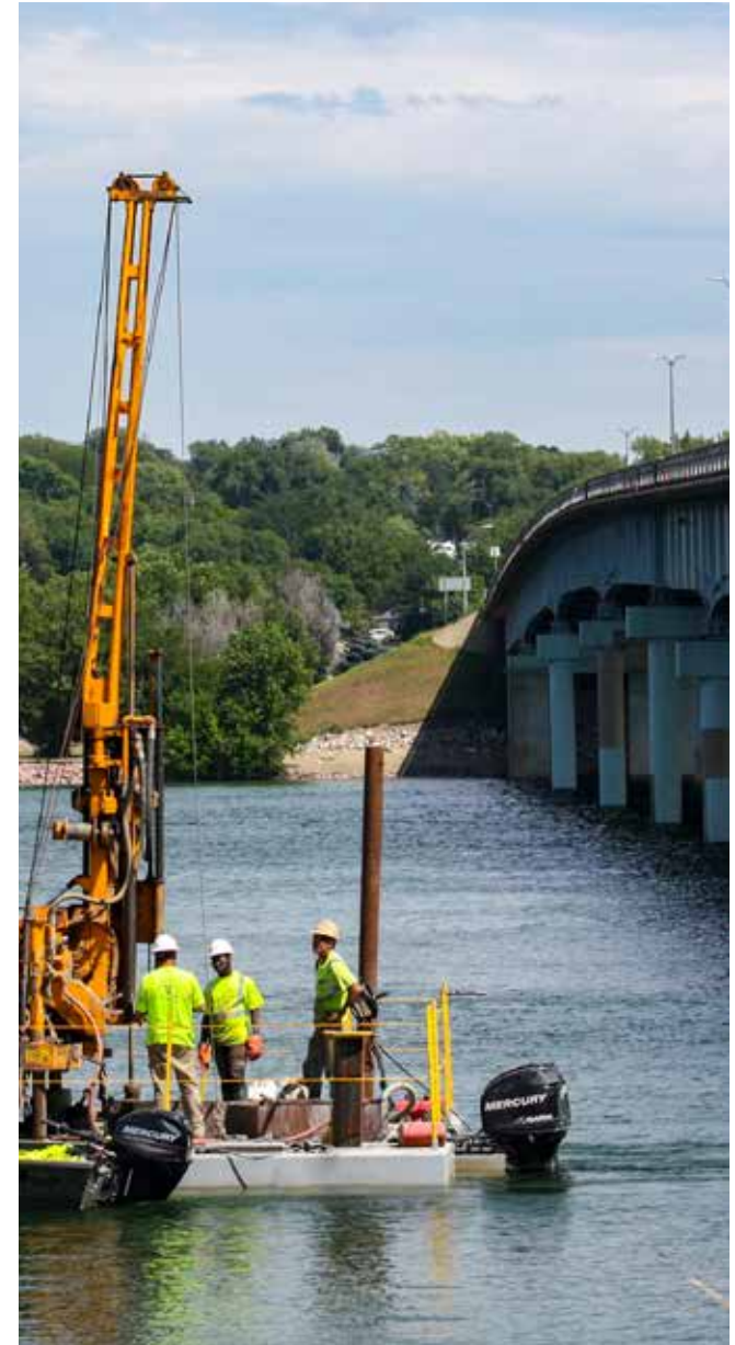
A geotechnical company hired by the SDDOT collects underwater data at the pier locations of the new Pierre-Fort Pierre bridge over the Missouri River in August 2018.
