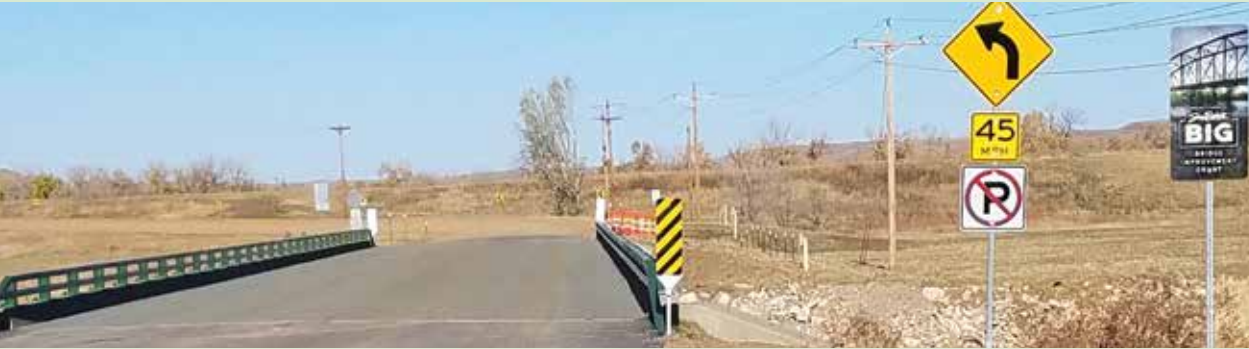
A recent polymer chip seal of this Meade County bridge deck and repainted railings will lengthen its service life. The bridge is on Alkali Road over the Belle Fourche River, three miles west of Hereford.
