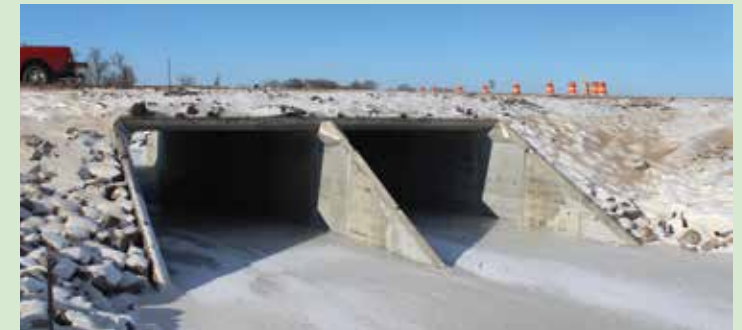
This new Grant County double-barrel box culvert is on 482nd Avenue over a creek. It is a half-mile south of Revillo.
