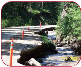
Improper Conveyance of Drainage
