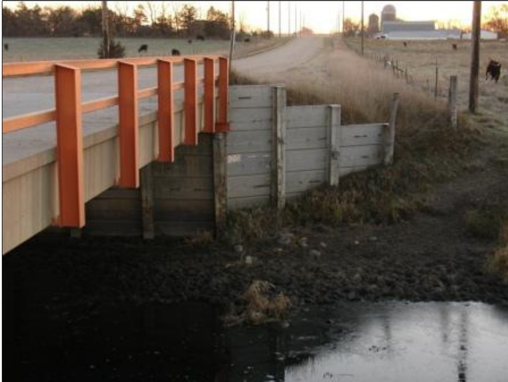
Photo 3 Downstream face of Willow Creek Bridge looking east along 20th Avenue South
